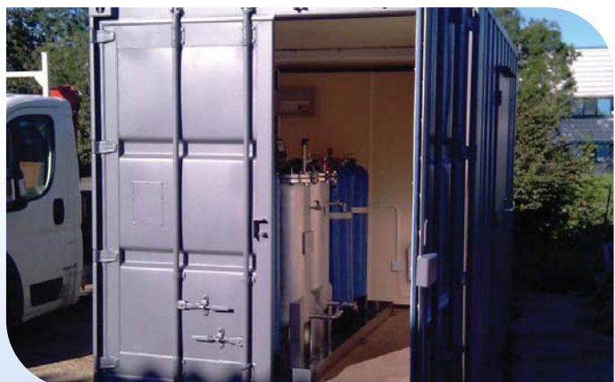
OPS Car Wash Water Treatment Unit installed in a 10ft Shipping Container
