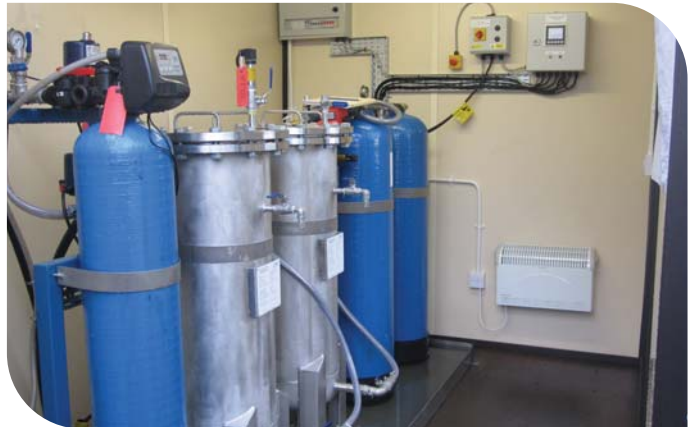
OPS Car Wash Water Treatment Unit
