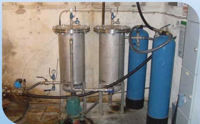
OPS Car Wash Water Treatment in the basement of a petrol station
