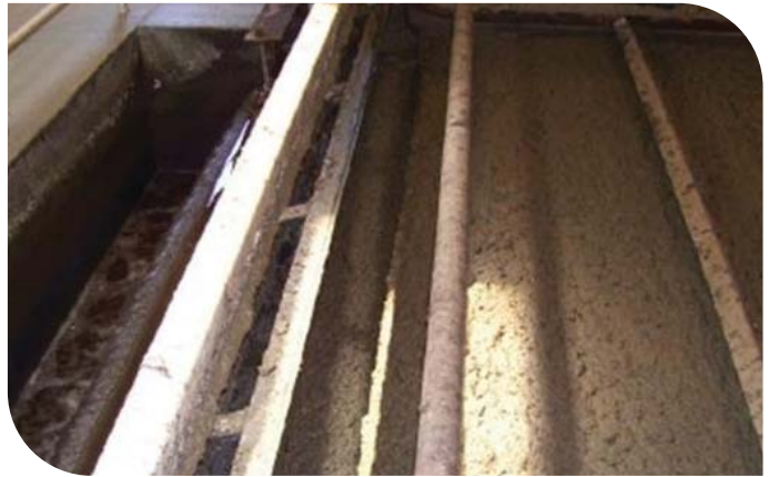
Foam on a DAF removed by a Scraper
