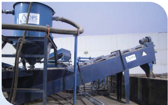
OPS Sand Cleaning Plant in Kuwait
